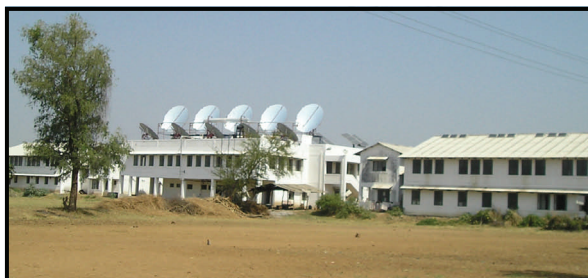
This Scheffler Community Steam Cooking System mounted on the rooftop of a school cooks 500 solar meals/day for students and faculty
